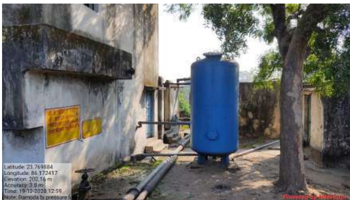
FILTER PLANT IN THE MINE AREA
